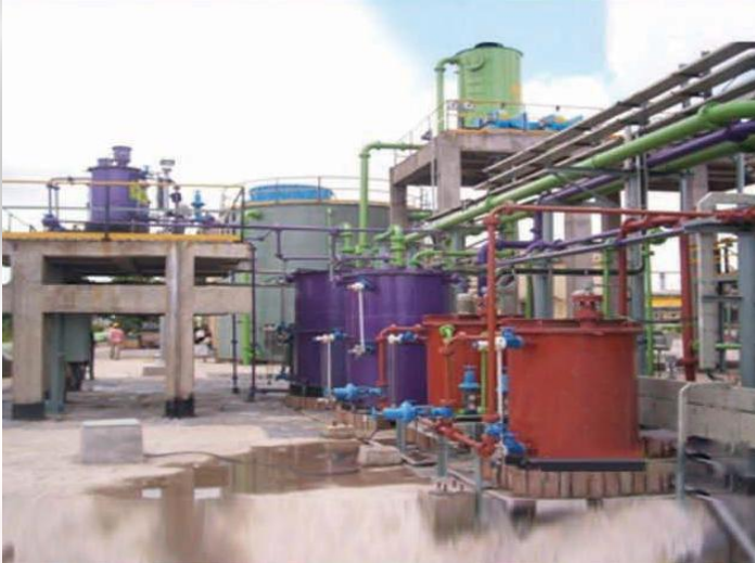
Effluent Treatment Plants
