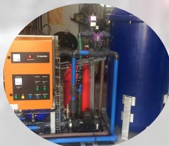
Raw Water Treatment and clarification Systems
